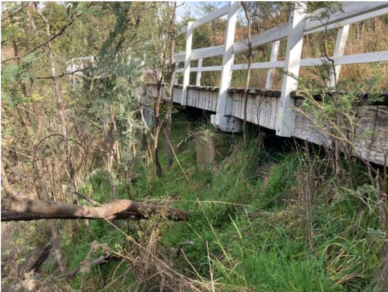
Photos 4 & 5: Existing concrete footings where bolting direct into rock was not feasible
