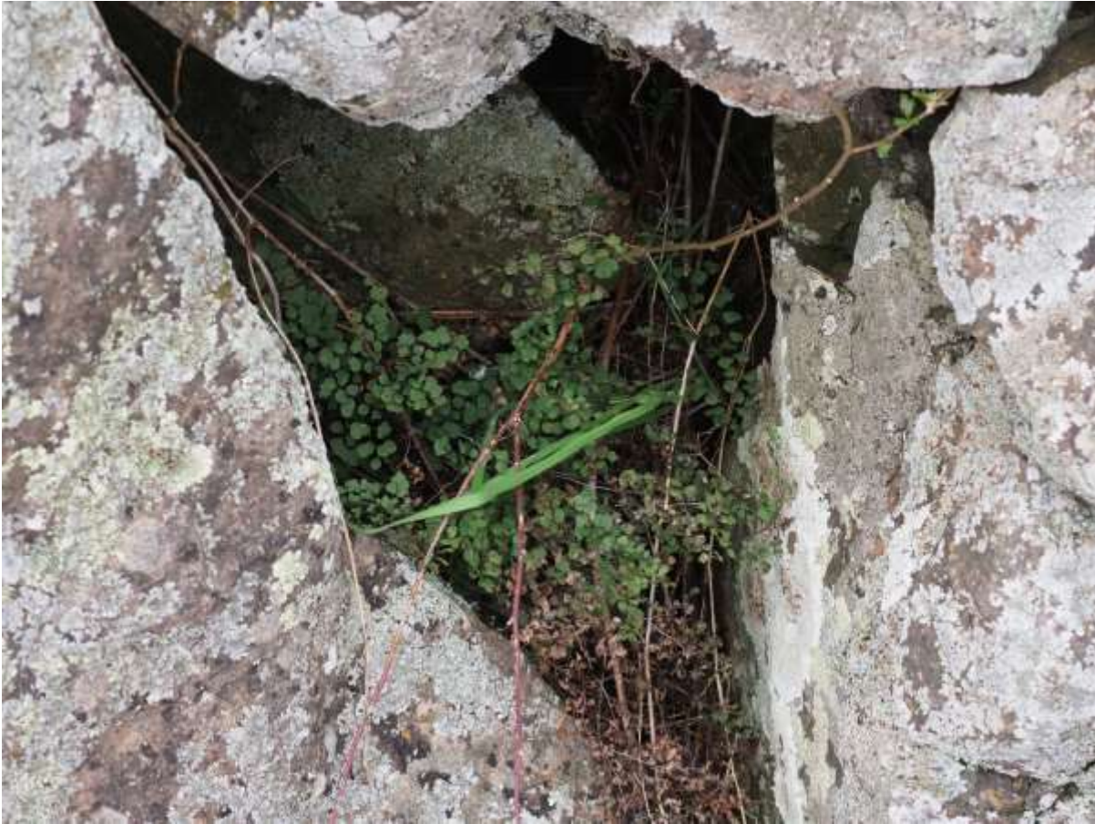
Photos 11 and 12 – maidenhair fern in a different part of the bridge also located at bridge level. A closeup of fern (top) and a photo of the same (below) showing its proximity to the edge of the bridge.
